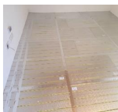
The room after the cable Line™T10 installation
